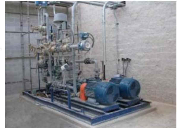
High Pressure Pumps
